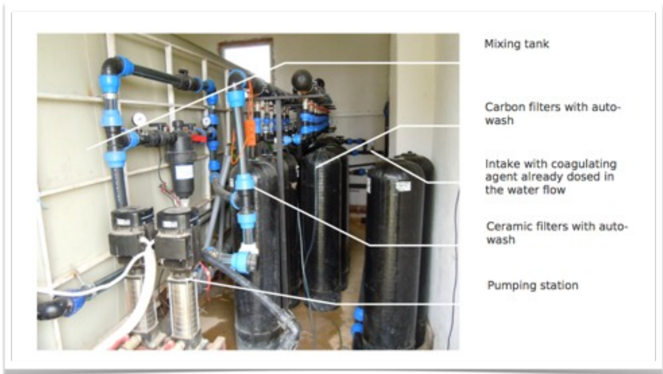
Real picture from a village water station modified for removing Arsenic from water (source water well). Picture taken while plant was under annual maintenance and active elements replacing.
