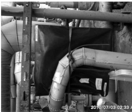
Image of insulated pipe at 460°C
