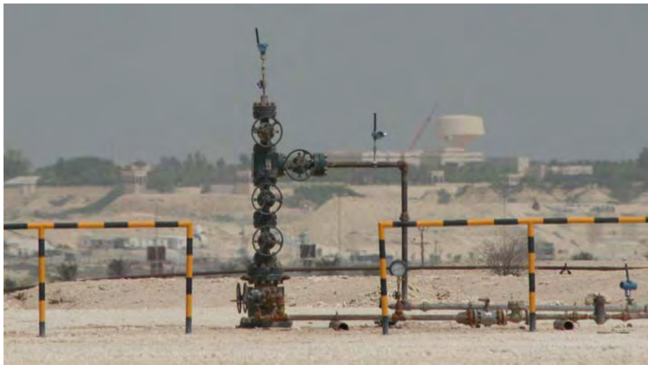
Remote pumps communicate wirelessly to a WirelessHART gateway. These Middle-Eastern pumps need performance monitoring so that engineers can make informed maintenance decisions. The gateway connects to the main control system over a WAN so that the engineers gain essential data at their desks. Installing wireless sensors on remote wellheads and other similar applications is much less expensive than hard-wiring.
