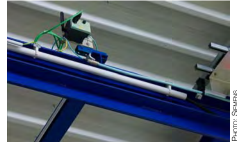
Fig. 1. With their IP65 enclosures the access points are installed freely in the field and connected directly to the RCoax leaky feeder cable (blue).
